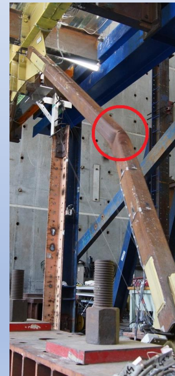
Overall Column/Brace Buckling Axial Load
